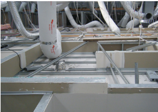
Figure 65: Unbraced partitions and service ducts.
