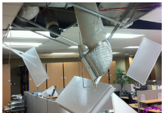
Damage caused by unrestrained ducting.
