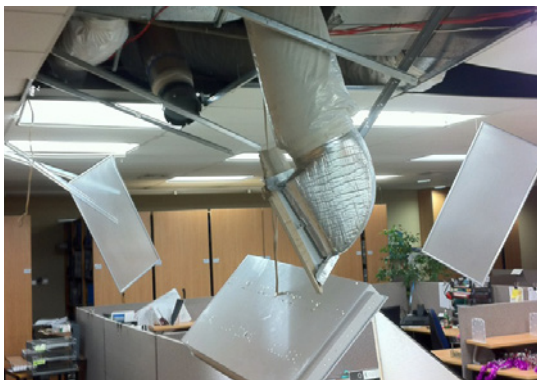
Figure 69: Damage caused by unrestrained services.
