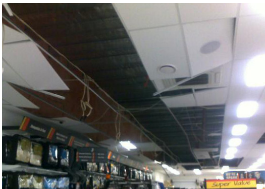
The result of an unbraced ceiling.
