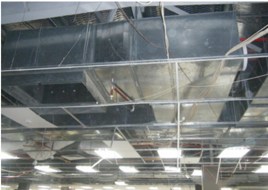
Figure 64: Lack of suspension points and service clearance.
