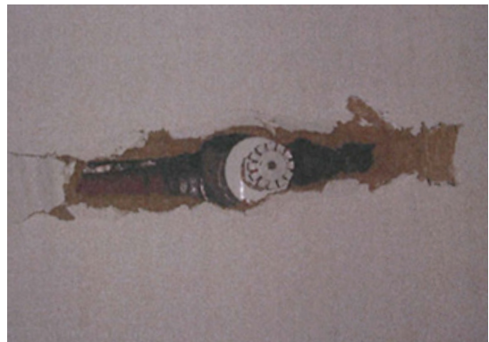
Damage from unrestrained fire protection system.
