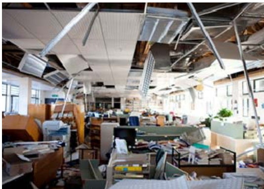
Damage caused by unrestrained services.
