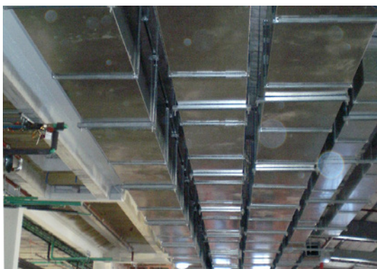
Figure 70: Lack of suspension points.
