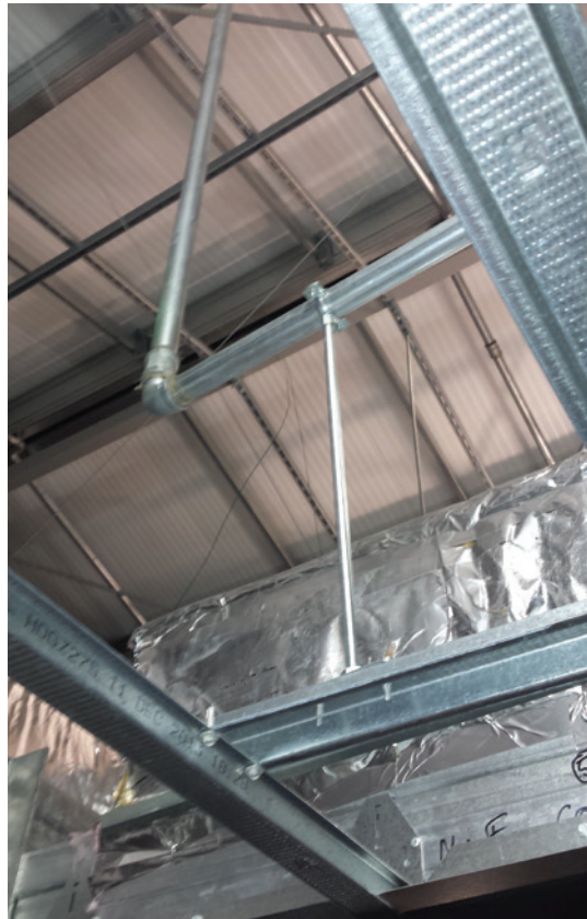
Figure 66: Sprinkler system supported from ceiling componentry rather than suspended from the building structure.
