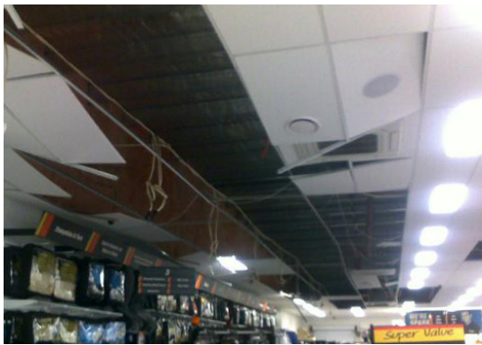
Figure 67: The result of an unbraced ceiling.
