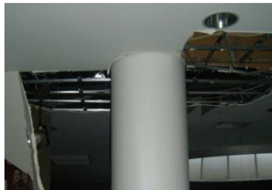
Plasterboard ceiling damage caused by interaction with structural circular columns.
