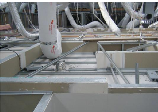
Figure 79: Unbraced partitions and service ducts.
