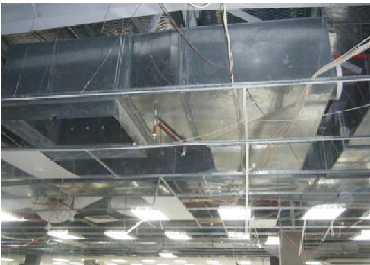
Figure 78: Lack of suspension points and service clearance.
