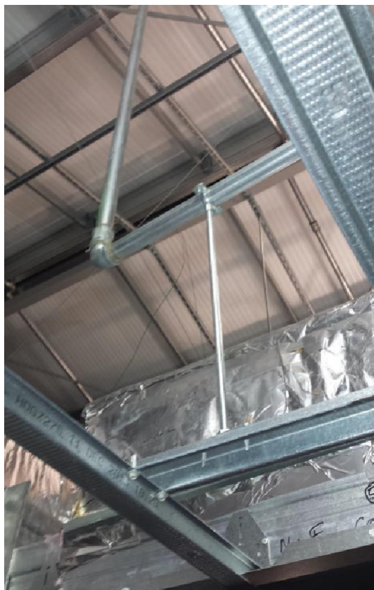
Figure 80: Sprinkler system supported from ceiling componentry rather than suspended from the building structure.
