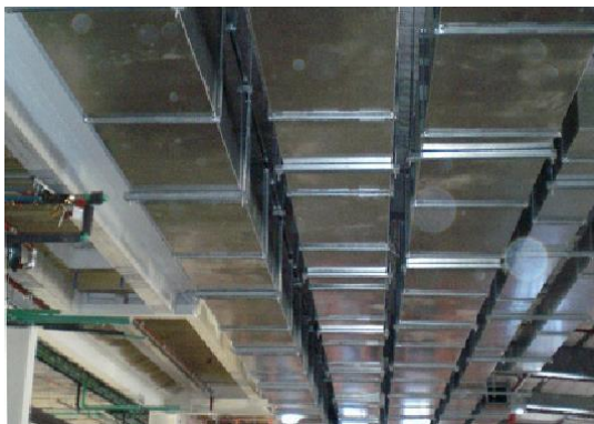
Figure 84: Lack of suspension points.
