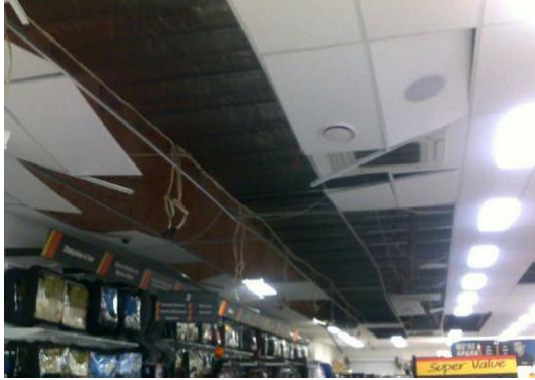
Figure 81: The result of an unbraced ceiling.
