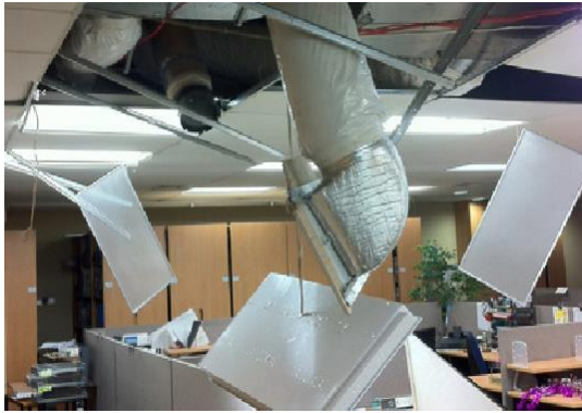
Figure 83: Damage caused by unrestrained services.
