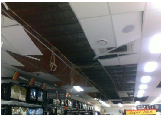
The result of an unbraced ceiling.
