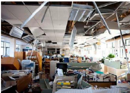
Damage caused by unrestrained services.
